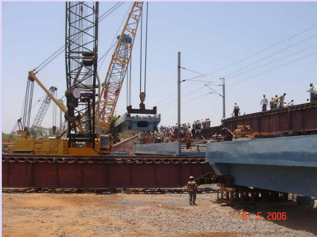
3 rd stage – Launching of PSC box girder in progress and is in final stage.
