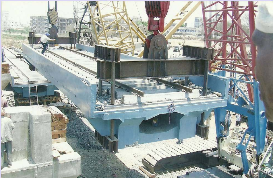
2 nd stage – PSC box girder weighing about 220 M.T. being lifted using 2 Nos. 400 M.T. capacity cranes from the ground level.
