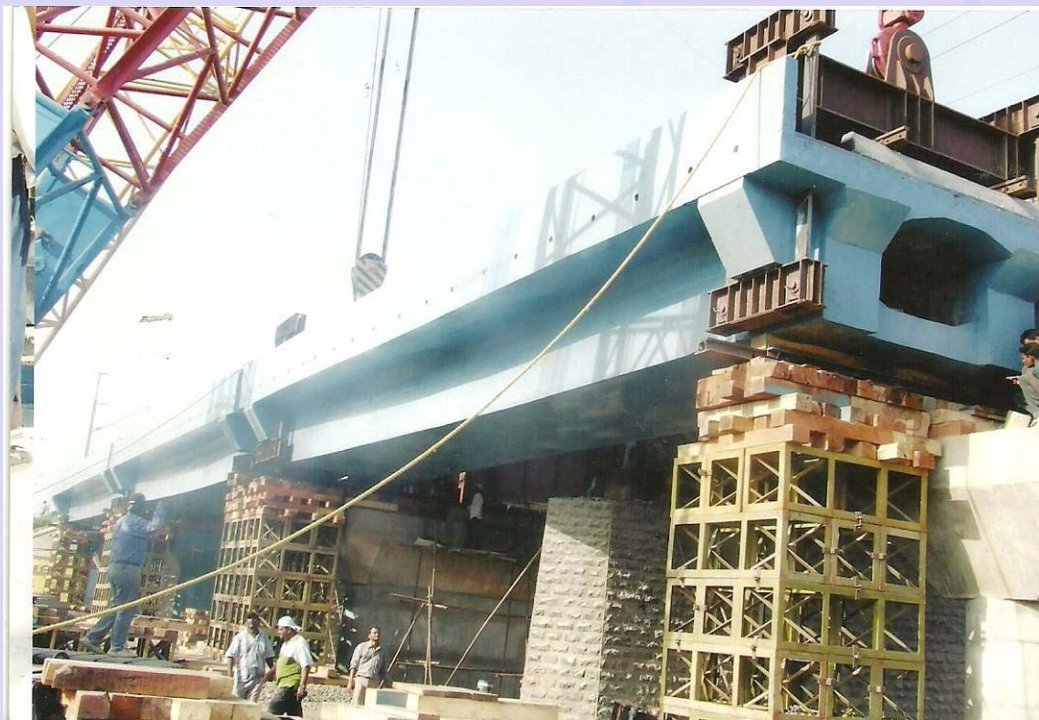
4 th & final stage – View showing PSC box girder placed on Temporary c.c. cribs before finally placing in position on new pier caps.
