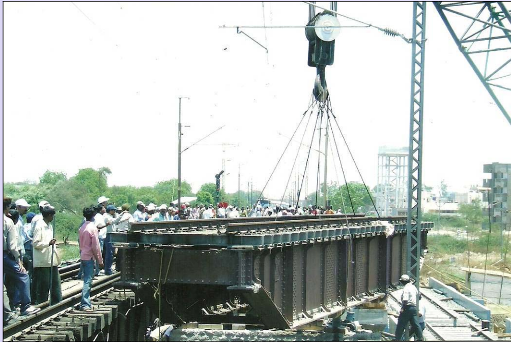
1 st Stage - 35 M.T. existing steel girder was de-launched by 400 M.T. capacity hydraulic crane.
